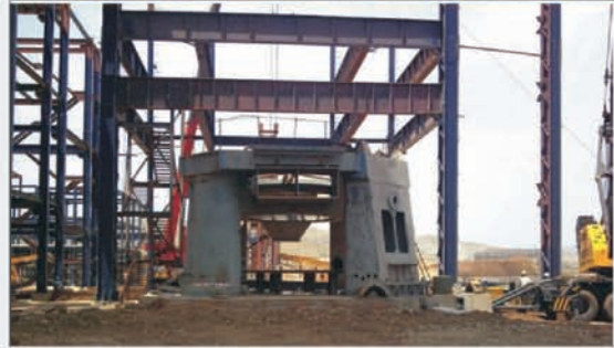
Fabrication and Erection works of Structural, Technological Structural and Equipment Erection of Cement Plant for Jindal Cement Works, Bellary in 2009
