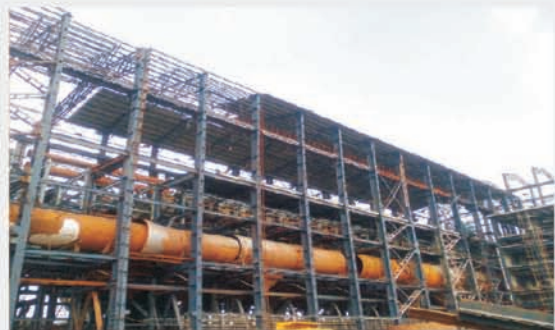
Fabrication and Erection works of Structural, Technological Structural Chimney, ESP and Equipment Erection of Sinter Plant 6500 MT for Jindal Steel Works, Bellary, Karnataka in 2005-07
